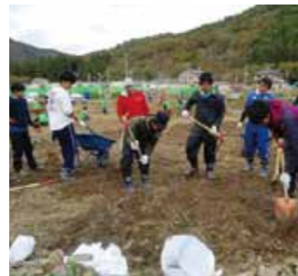
Leveling of land Countless stones come out thick and fast in the digging. Volunteers interact with residents of temporary housing.
