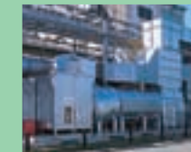
■ Heat cycle exhaust treatment system
