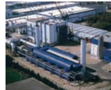
Heat accumulating deodorizing furnace at Nitto Europe N. V. (Belgium)
