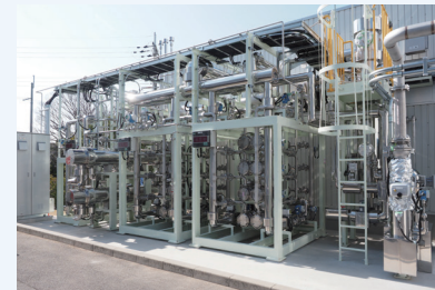
The demonstration unit in service at the Shiga Plant
