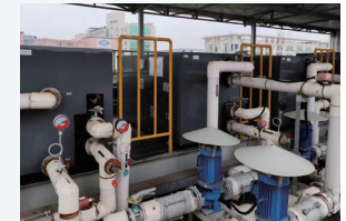
Heat pump system
