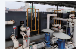
Heat pump system
