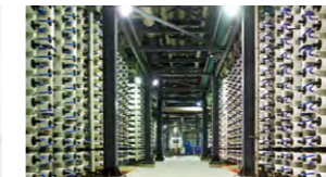
Example application of membrane treatment technology—recovering liquid discharge from production processes
