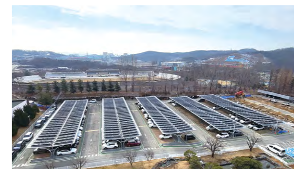
Solar carport at Korea Nitto Optical
