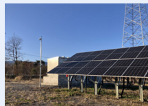
Solar Power Generation System Located Outside Nitto's Premises
